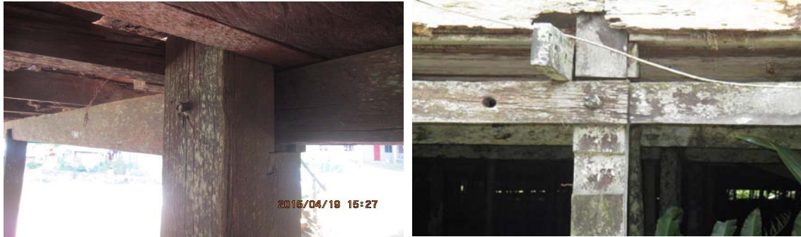
Fig. 4. Mortise and tenon connection of timber post and beam strengthen with steel or timber peg.
