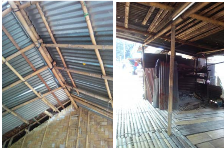
Fig. 6. Bamboo for ridge board, rafters and purlins of a roof structure tied with rattan and polymer cable.
