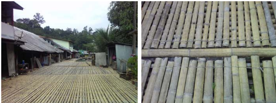
Fig. 5. Split bamboo tied to the bamboo joist (underneath) with rattan for floor construction.
