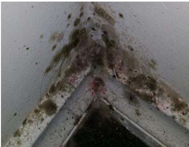
Fig. 9. Mould growth in carpet, wall base, skirting board and on plasterboard
