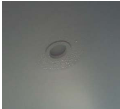
Fig. 2. Condensation forming around downlights
