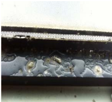
Fig. 1. Excessive condensation and mould on aluminium window
