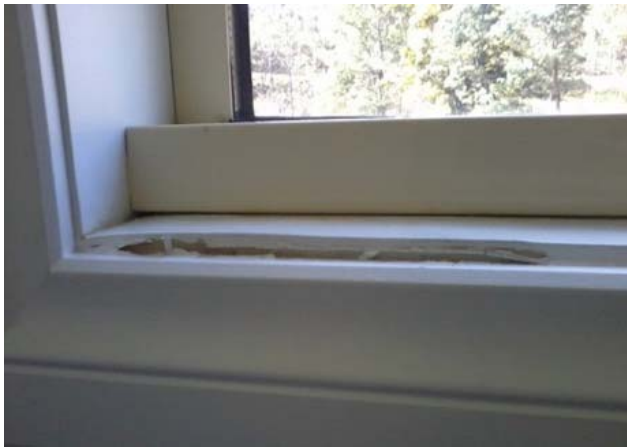
Fig. 7. Expansion and cracking of timber due to moisture pooling at glazing
