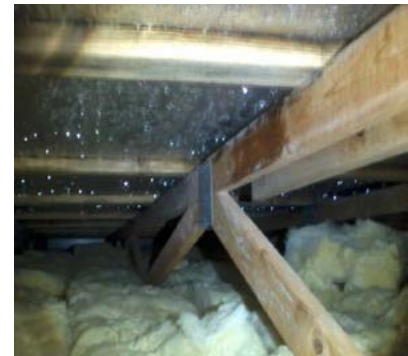
Fig. 3. Condensation forming in roof space
