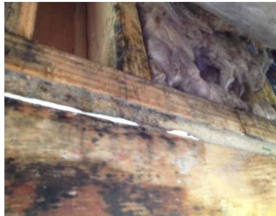
Fig. 8. Mould growth on bearer, joist, wall batts and gaps left in wall insulation
