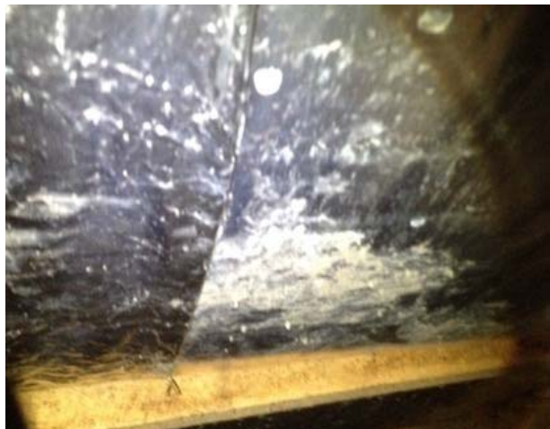
Fig. 10. Mould growth on foil backed blanket sarking system
